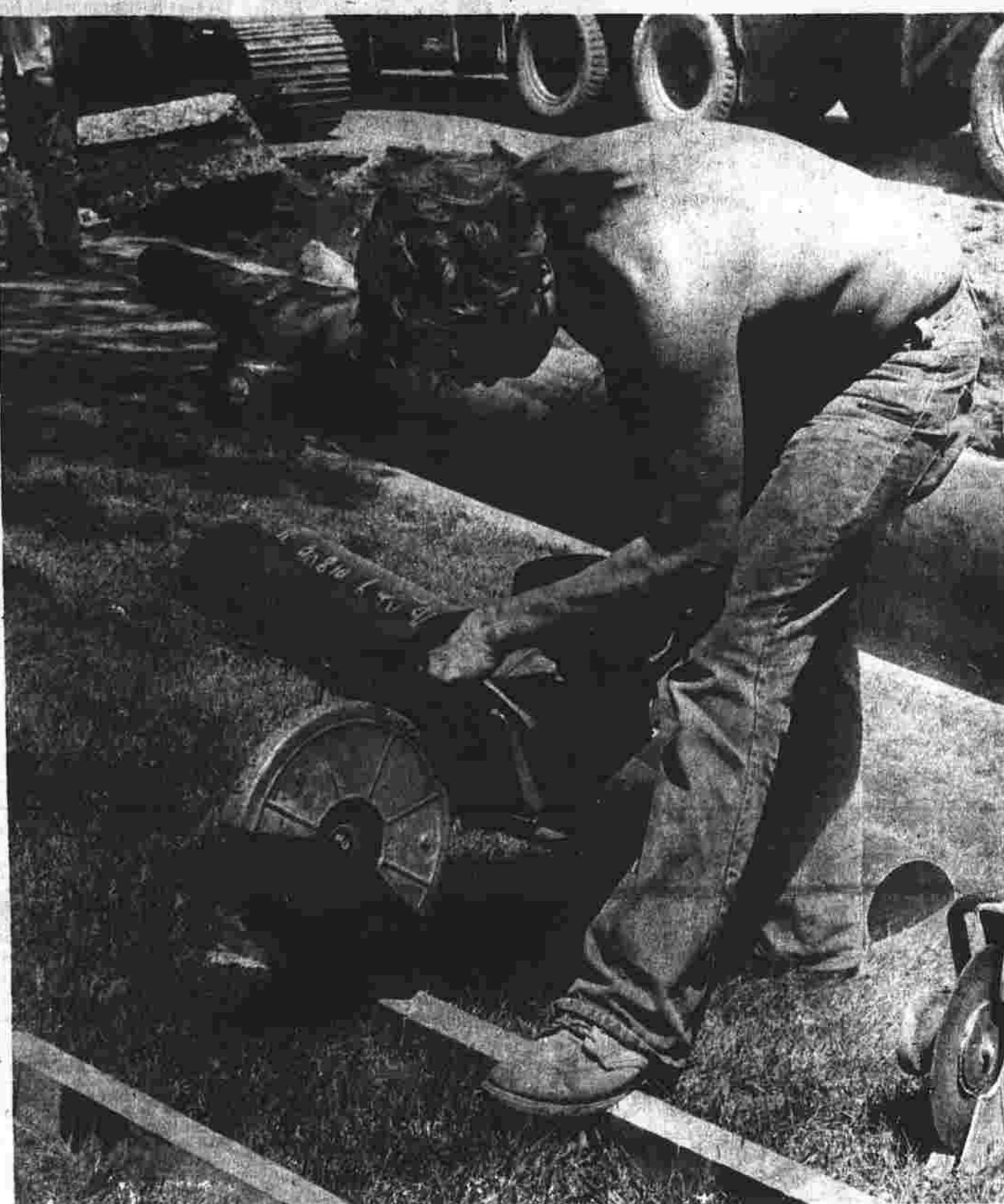
A new main... Jim Dannick of the Schultz Construction Co. labors in the afternoon heat on Main Street near St. Bridget Church where workers are installing a new water main. (Herald photo by Pinto)
